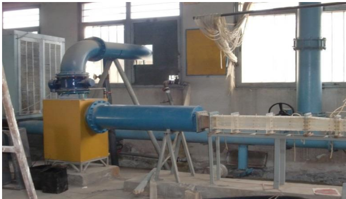
Fig. 1. A view of the supply tank of head (Hosseini et al.)
