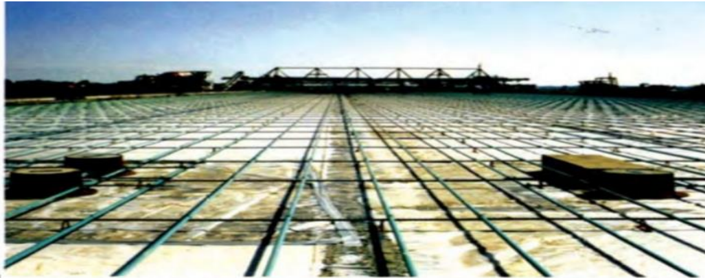
1200-ft-long post-tensioning tendons ready for concrete from the bridge deck paver in the distance.
